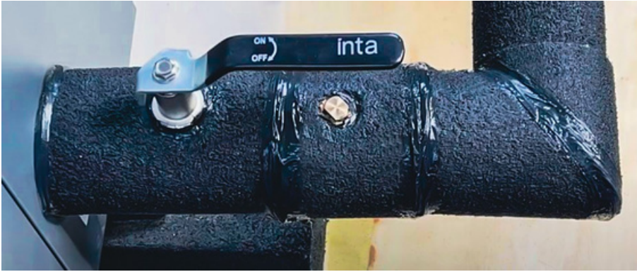
Sealing of isolation valve, antifreeze valve, 90° elbow and bonding to heat pump.
